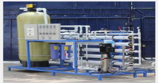
Fig. 6. Nanomembrane filtration plant
